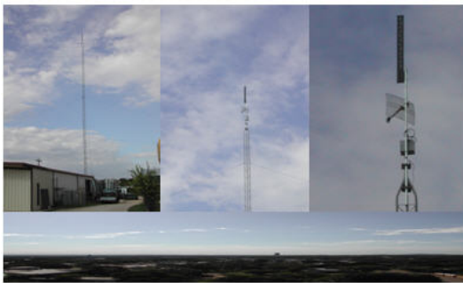
Base Station for Bandera Site
